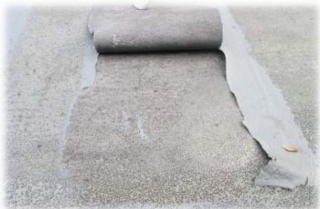
Pull free end. Should the coating be freely removed from the substrate then a primer should be considered and re tested.
