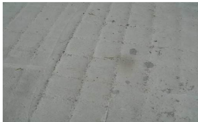
Example of 'reinforcement ripple'
