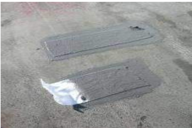
Embed a strip of polyester fabric into the roof coating and allow to cure completely
