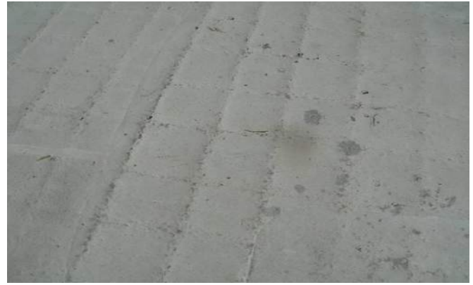
Example of 'reinforcement ripple'
