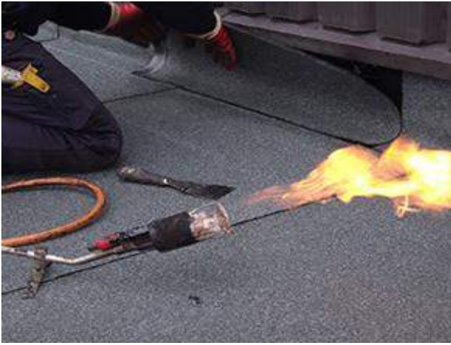
Gas torch unsupervised and abutment to cladding
