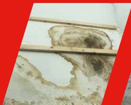
Dampness or mould on ceilings and walls
