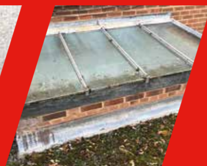
Damaged or fragile roof lights
