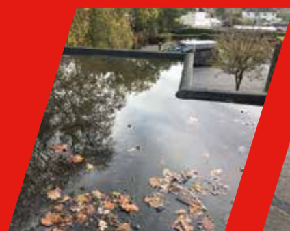
Ponding or standing water
