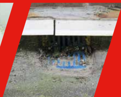
Blocked drains and gutters
