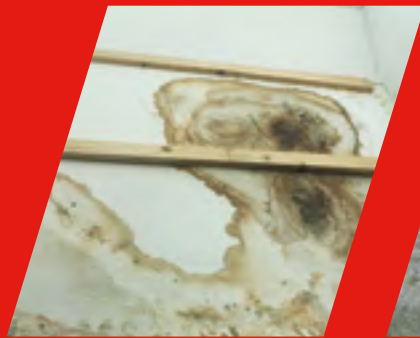
Dampness or mould on ceilings and walls
