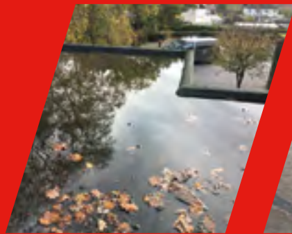
Ponding or standing water
