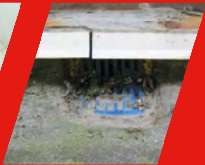
Blocked drains and gutters
