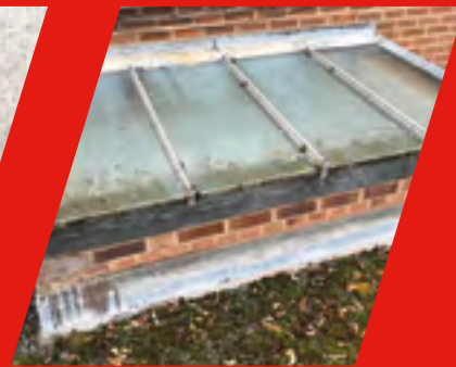
Damaged or fragile roof lights
