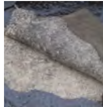
Failed peel test - easily pulled from the substrate
